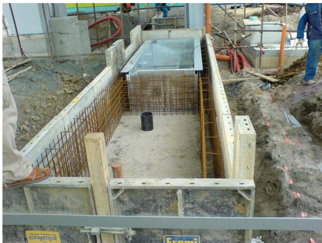
Settled blocker + second plate with drainage pipe
